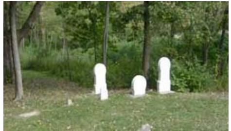
The Venetian marble stones belonging to the Pickering family were cleaned and repaired.
