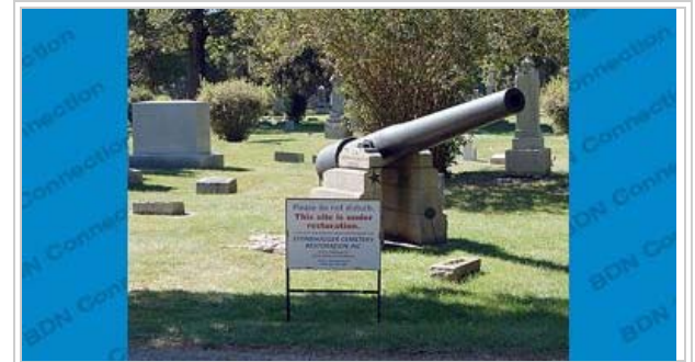
A sign placed by Stonehuggers Cemetery Restoration in the Rockton Township Cemetery notes work is in progress to restore headstones. Work began Monday to restore and repair headstones.
